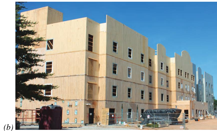
Figure 1-6: Platform-type construction: (a) Stadthaus (Photo credit Will Pryce); and (b) Redstone Arsenal (Photo credit Lendlease)
